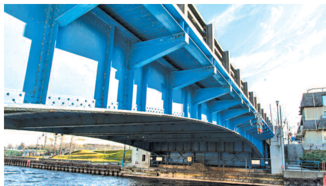
Work is set to begin next week on a $1.9 million project to repair and upgrade the bascule bridge as it spans the Pine River Channel along U.S. 31 in downtown Charlevoix. The project is expected to take about six months to complete and will require overnight closures of the bridge for a period this spring. PHOTO BY SCOTT RICHARDS
